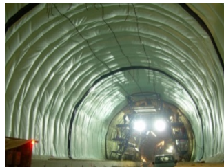
Figure 2: a) SC system installed
