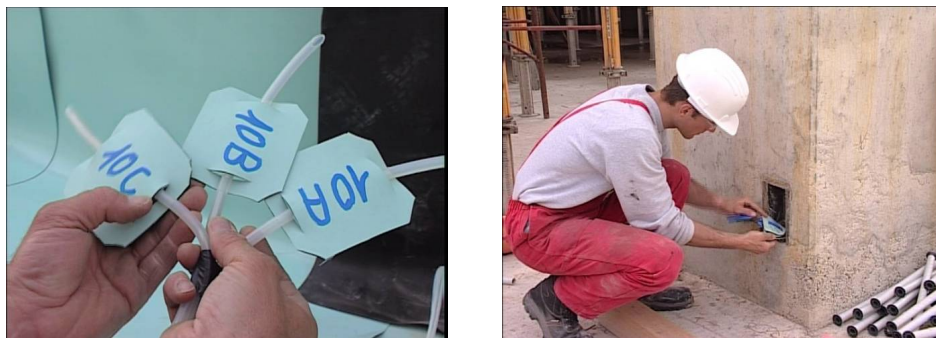
Figure 5: a) injection pipes numbered for each sector b) positioning of the box in the structure
